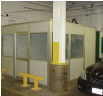
Modular walls were used in this previously used corner of this parking garage to create a clean, comfortable office space for security personnel.
